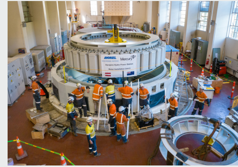
The crane delivering the rotor for Generator Two to its new stator windings.
